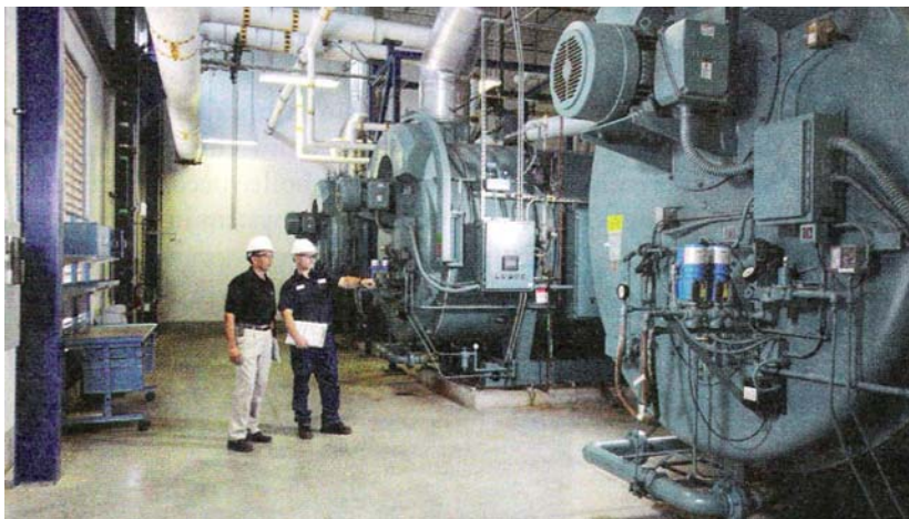
A system audit is a way to identify energy losses.
