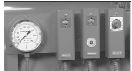
Figure 5-3 Hot Water Controls
