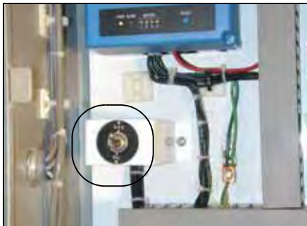
Figure 2-1 Gas/Oil Selector Switch
