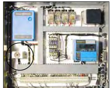
Figure 2-21 Control Panel with Gas/Oil Selector Switch
