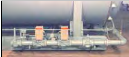
Figure 2-26 Main Gas Train
