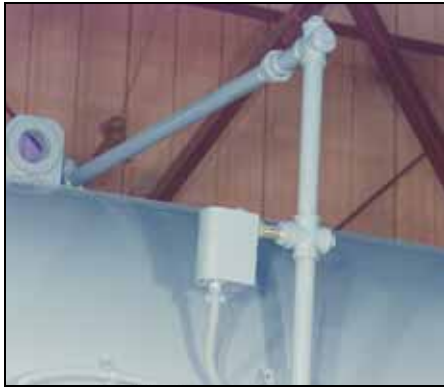
Figure 1-7 Auxiliary Low Water Cutoff
